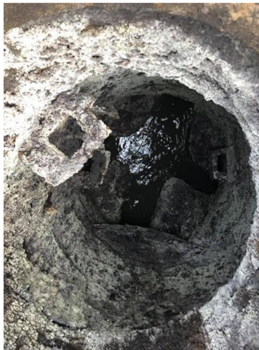
Fig. 1. Sulfate corrosion occurring in a sewer well
