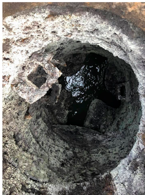
Figure 1. Heavily corroded manhole.
